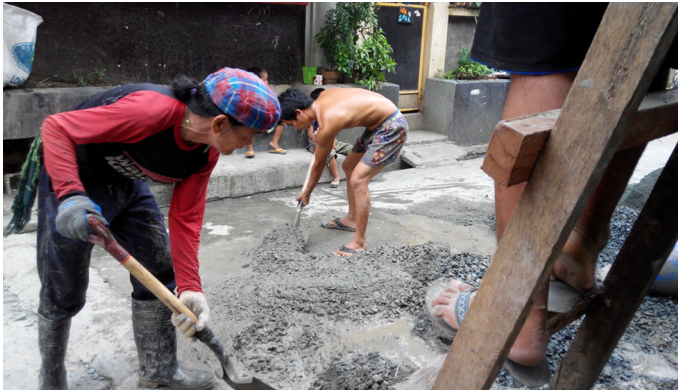
Fig. 4 “Both females and males are working on the construction of rebuilding together.” Taken and written by Francia, June 22, 2014
